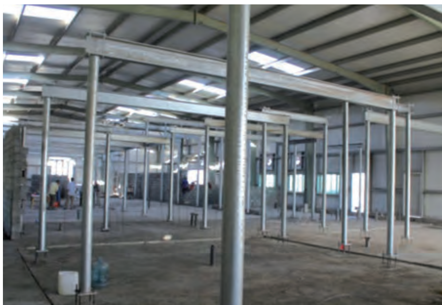
Travi e colonne in acciaio zincato, di sostegno guidovie Rail's supporting structure composed of hot galvanized beams and columns
