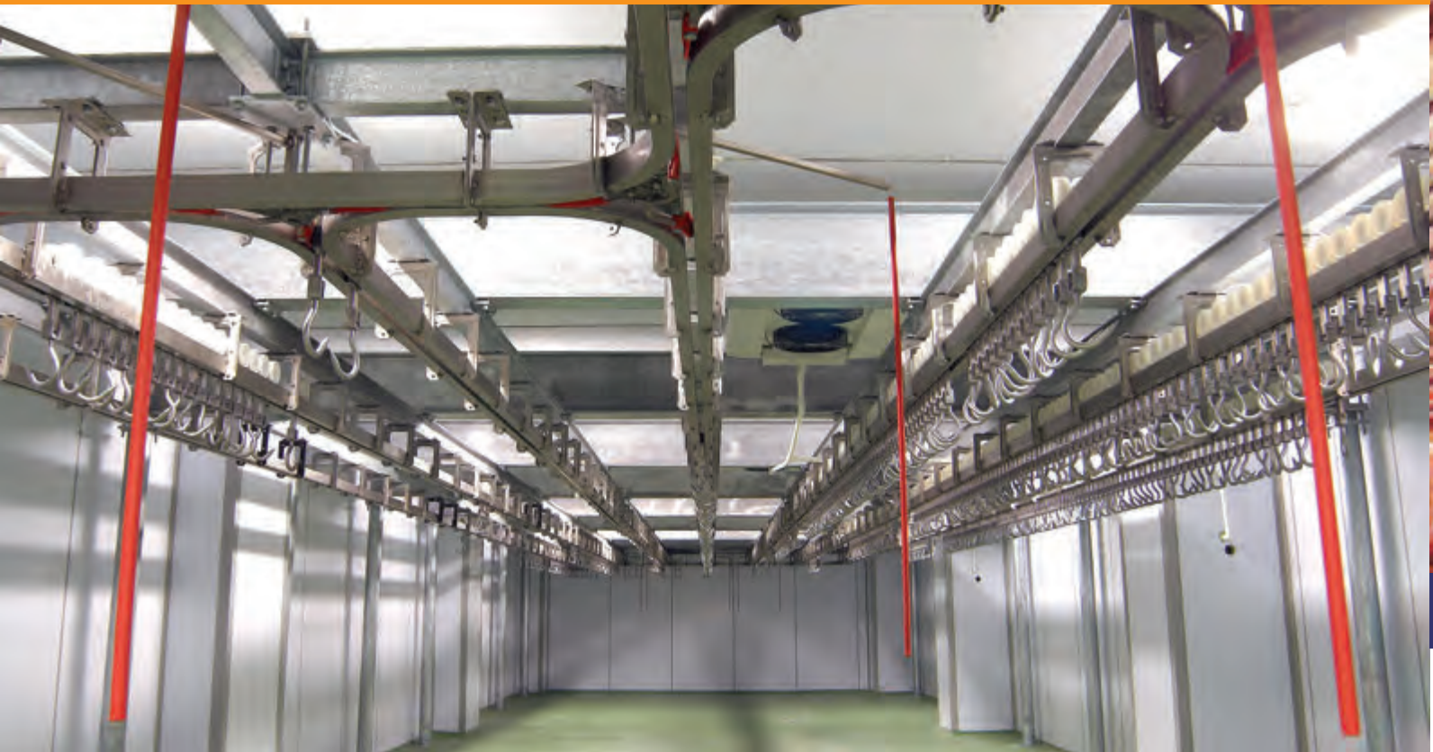
Cella frigorifera con guidovia in birotaia inox e struttura di sostegno Cold room equipped with stainless steel bi-rail and supporting steel structure
