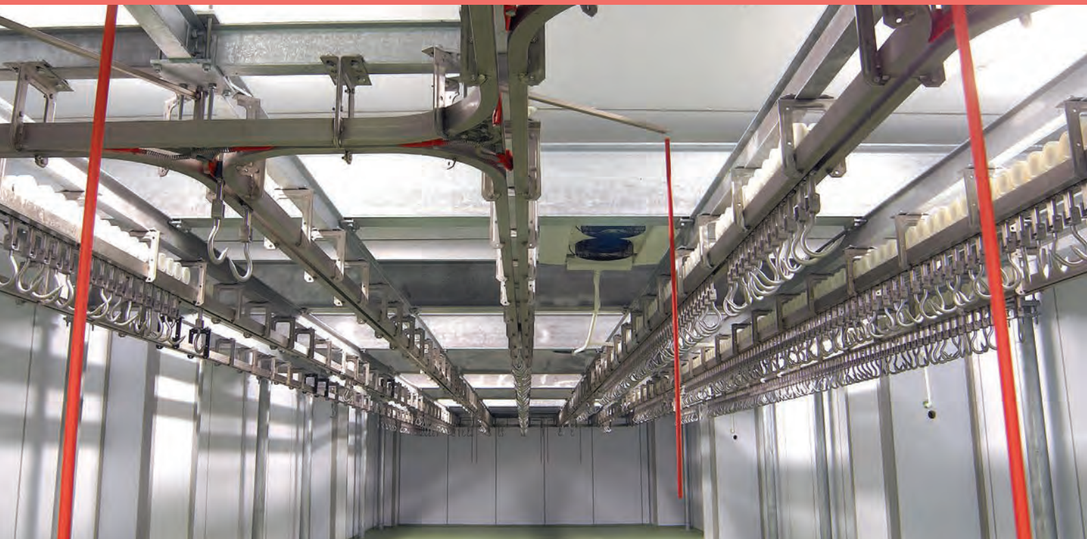
Cella frigorifera con guidovia in birotaia inox e struttura di sostegno Cold room equipped with stainless steel bi-rail and supporting steel structure
